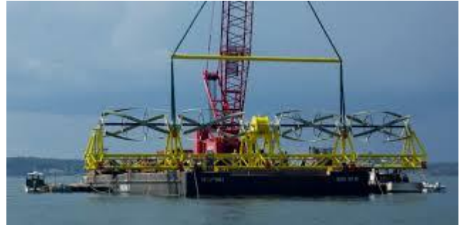
ORPC's TidGen tidal power unit being installed in Cobscook Bay, ME. Photo via ORPC.
